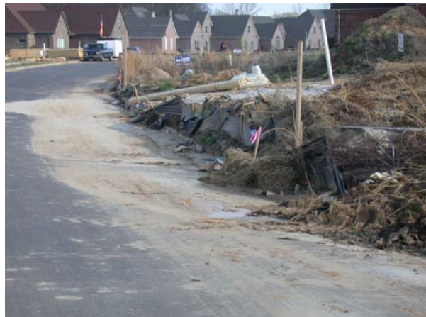
Bad management practice in subdivision on Oliver Creek (March 2004)
