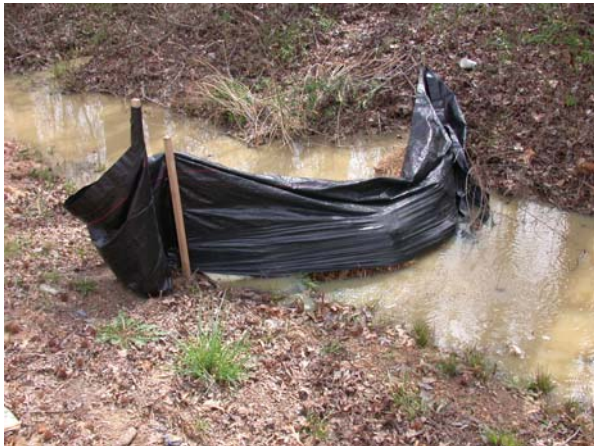
Poorly placed silt fence along water line construction along Hwy 70/79, near Lakeland City Hall (March 2004)
