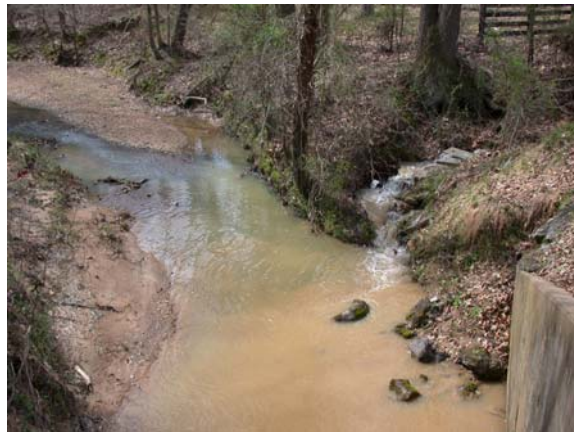
Discharge from water line construction adding sediment load to Scotts Creek. (March 2004)
