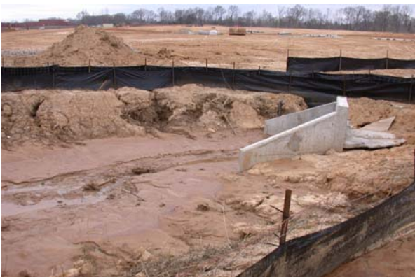
Construction at tributary to nearby Scotts Creek east of Oliver Creek. (March 2004)
